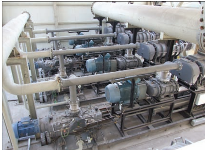
Degassing pumping modules made by Edwards and installed in a production facility.
